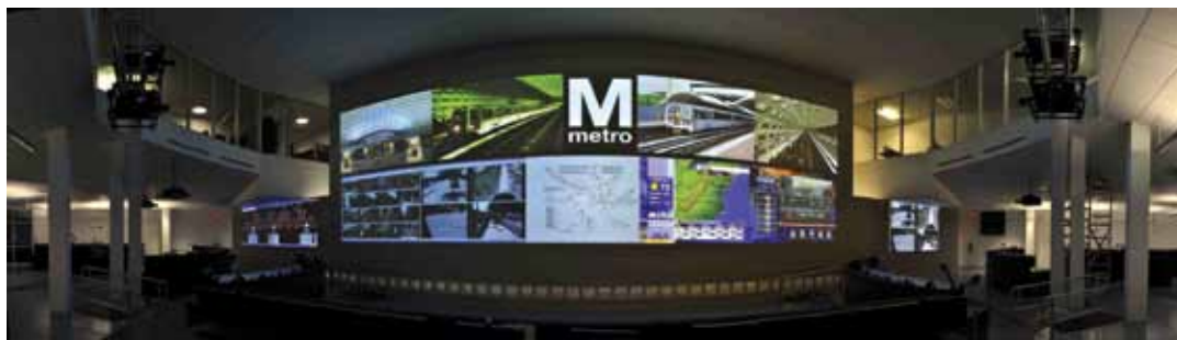
Washington Professional Systems integrated this command and control center for the Washington Metropolitan Area Transit Authority's rail operations.
